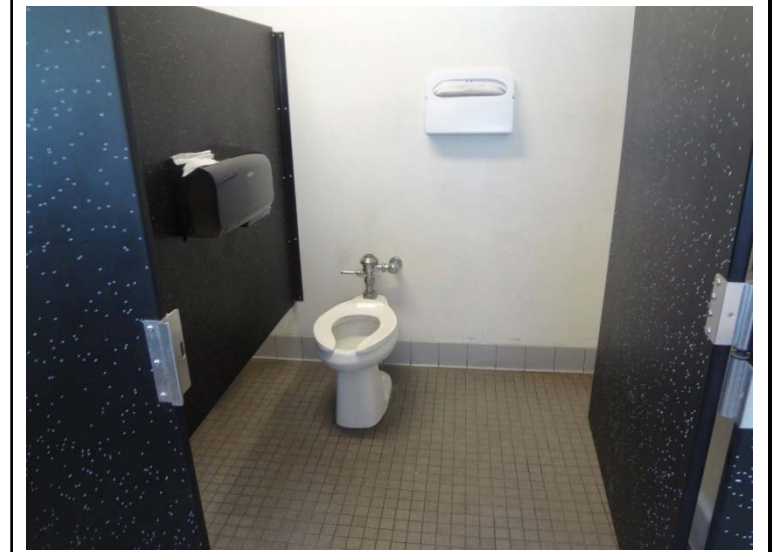
Photo -12 Building Number: 3 Accessible stall within building 3 requiring handrail.
