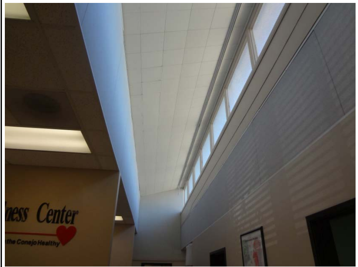
Photo -22 Building Number: 7 Ceiling condition and clerestory windows of medical training classrooms.
