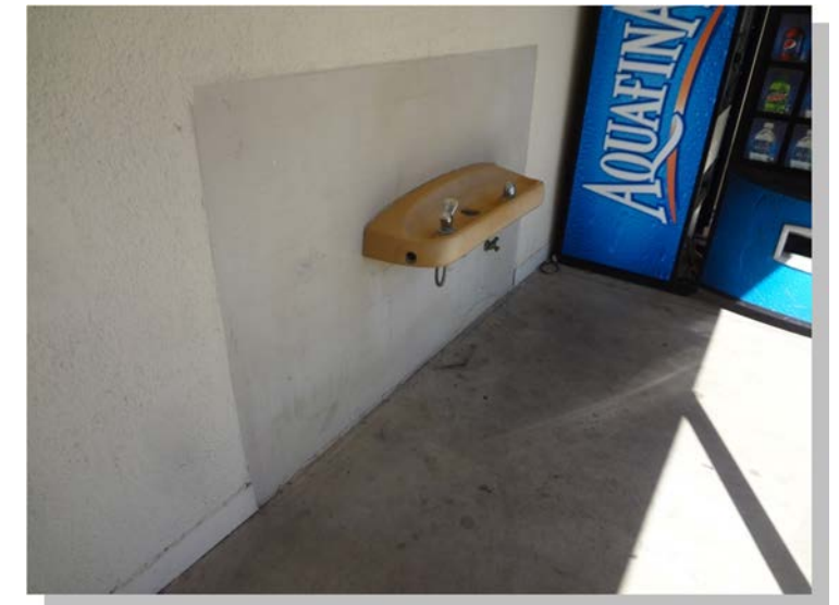
Photo -2 The drinking fountains have not been updated to current accessibility standards
