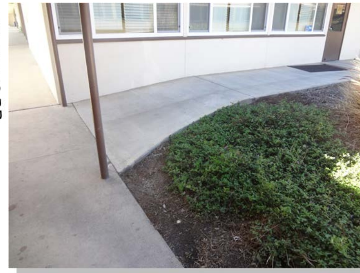
Photo -4 There are site accessibility issues all over campus that will need to be addressed when the school is modernized
